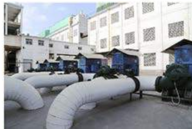
永煤集团循环水泵应用现场 (型号: 600S22 数量: 9台套) Yongmei Group circulation pump working site (Model :600S22, 9sets)
